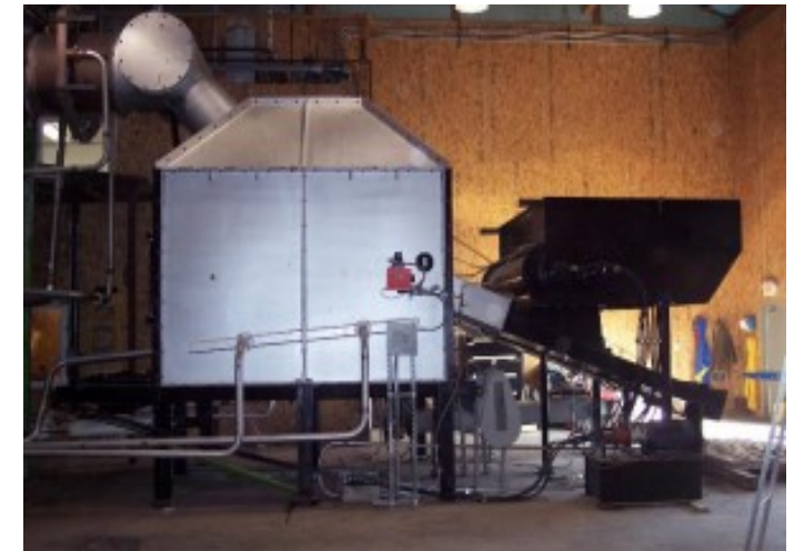
Fig.3. View of the gas generator in Coaltec Energy.
